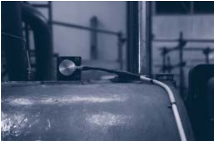
Pedestal vibration monitoring
