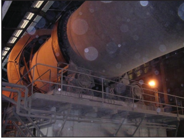
Kiln with support and drive structure
