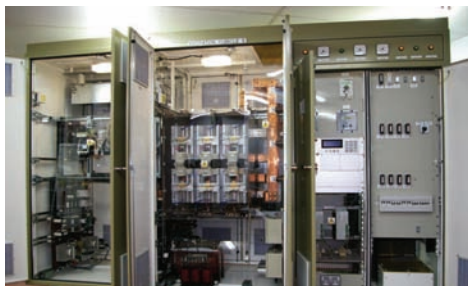
Control cabinet housing circuit breaker, thyristor racks, Microprocessor control system
